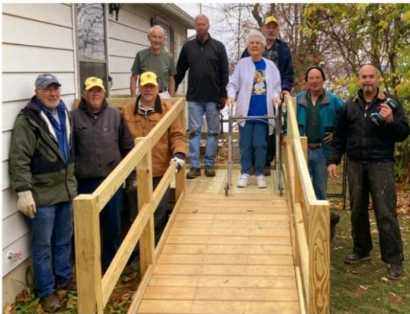
Lions who installed a ramp on November 13 at a home on Arrowhead Beach in Dresden: top row from left homeowner George Schleeauf, Norm Koek, Florence Schleeauf and Larry Strickland. Bottom from left Leigh Mackerchar, Rick Elliott, Dick Harper, Don Willmott and Chad Peek.
